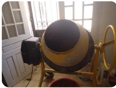
Figure II.11: Malaxeur a Béton
