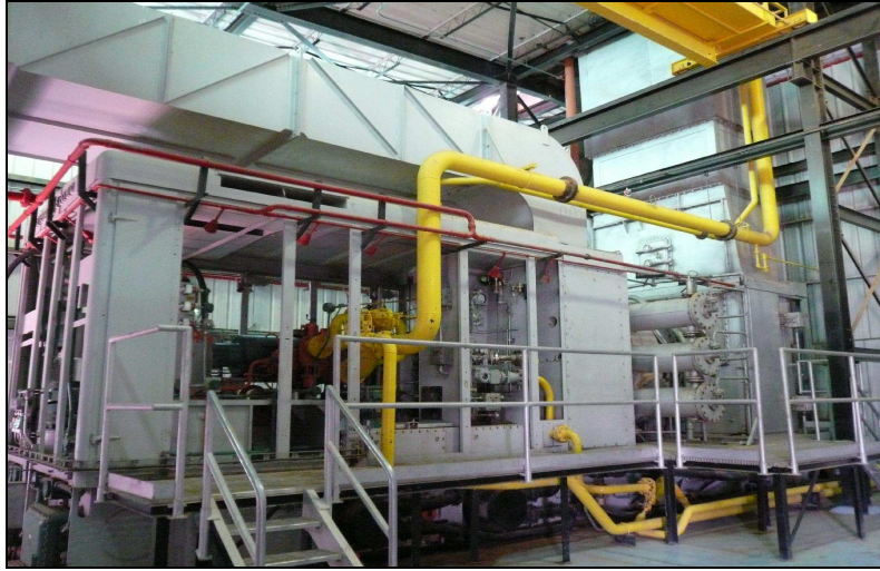
Figure II.9: Turbine à gaz GE MS3002
