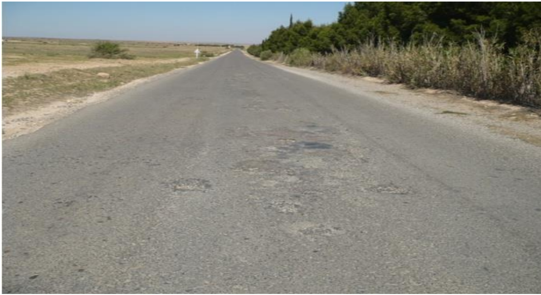
Figure III.4 : PK 06+400 (Epaufures + arrachement)
