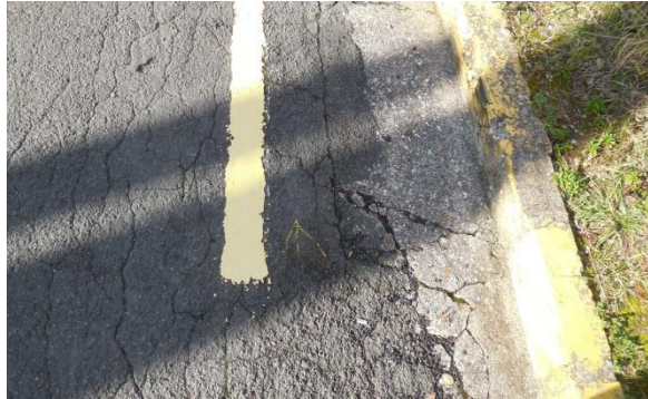
(b) Ramification des fissures
