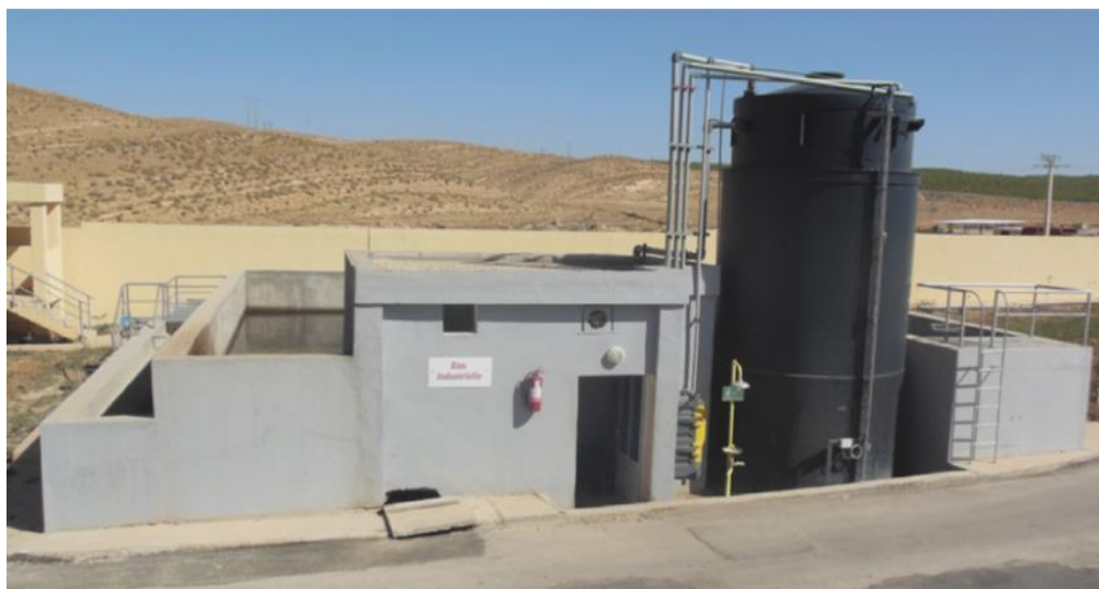
Figure III.16 : Station de chloration nouvelle file
