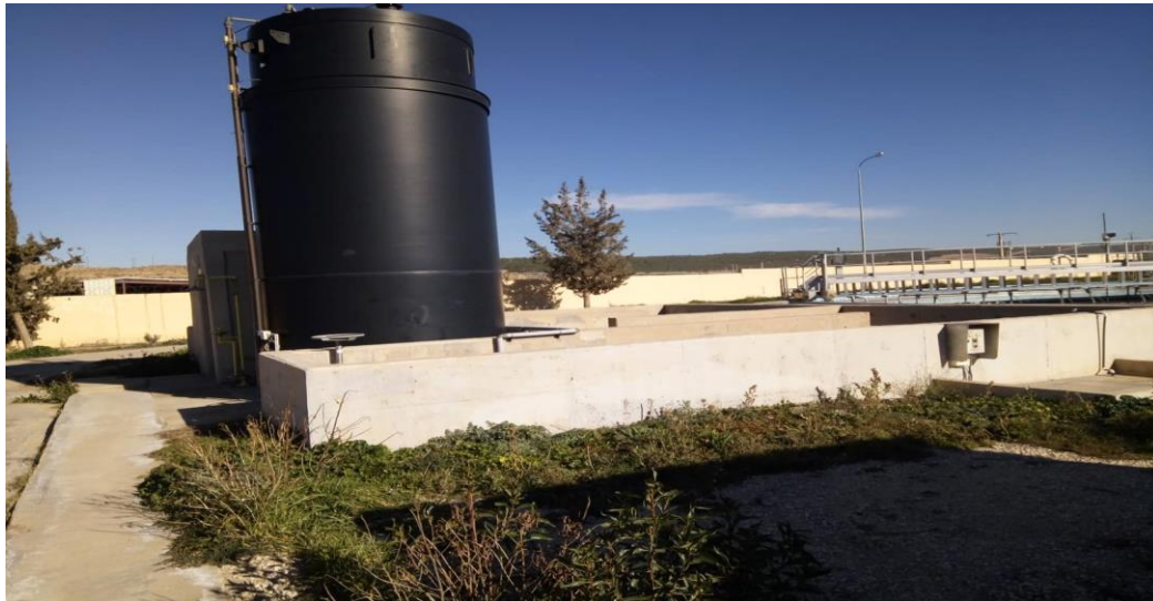
Figure III.12 : Station de chloration file existante
