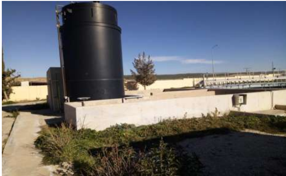
Figure IV.11 : Station de chloration file existante
