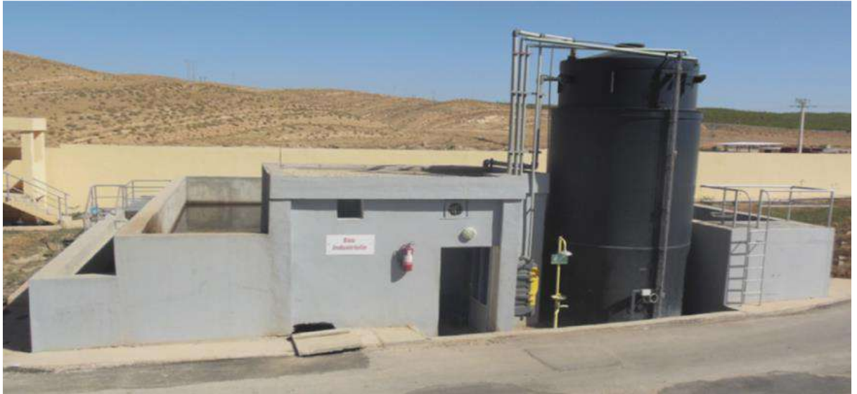
Figure IV.15: Station de chloration nouvelle file
