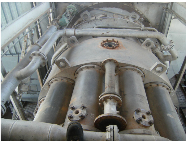
Figure B.1: Combustion chambers of GE Gas turbine 5002C
