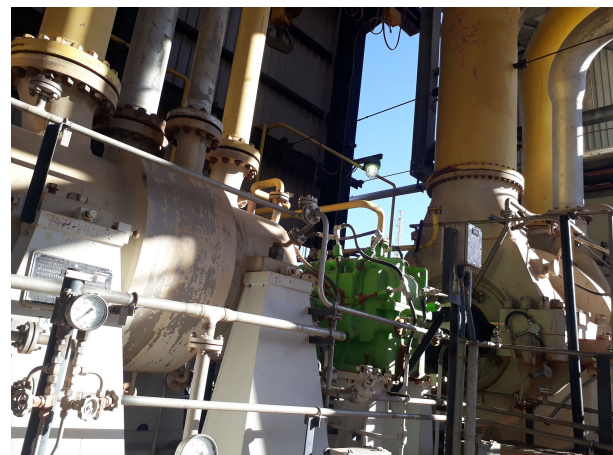
Figure B.2: HP and LP of centrifugal gas compressor
