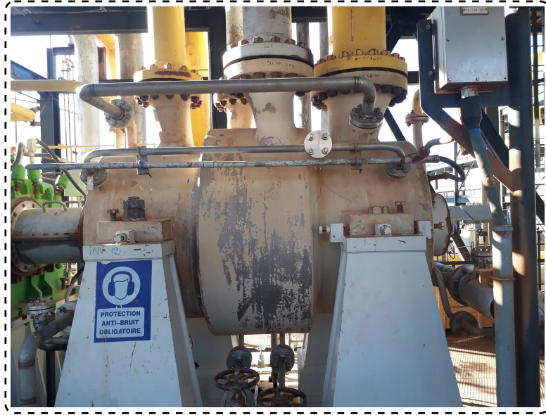
Figure 3.4: The studied centrifugal gas compressor system BCL 505 installed in the natural gas compression station
